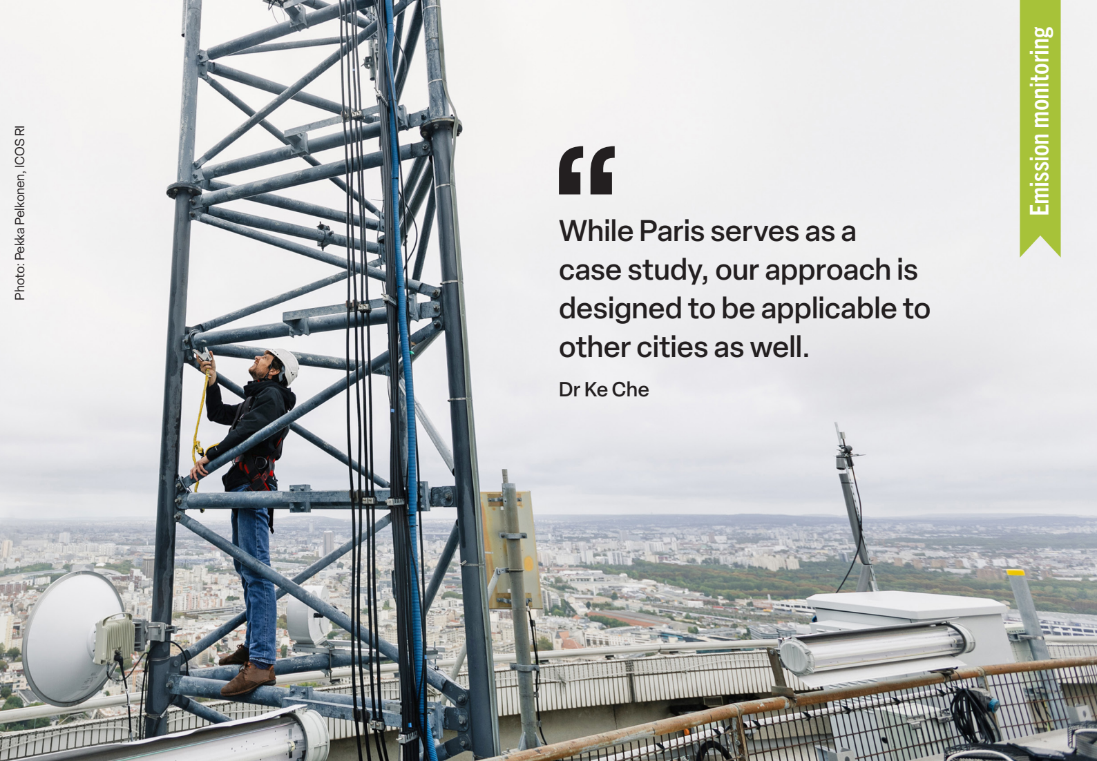
Monitoring equipment installed on the 128 metre Romainville tower in Paris.
